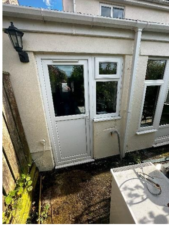
Pic16: DPC breached
