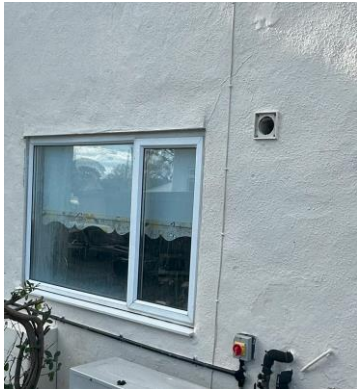
Pic13: Cracking above window head
