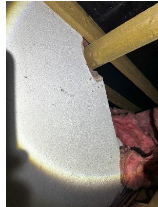
Pic28: potential lack of support to perlin
