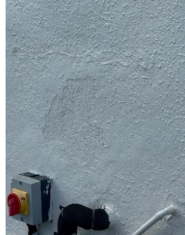
Pic18: Damaged render
