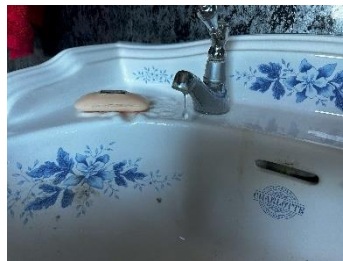
Pic41: leaking tap
