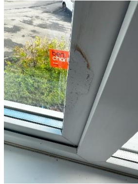
Pic20: Damaged frame
