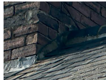
Pic 7: missing lead work saddle
