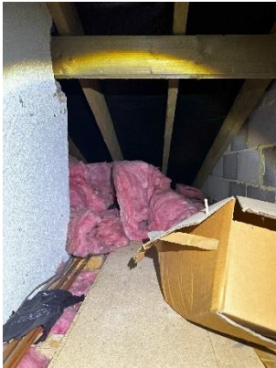
Pic26: displaced insulation
