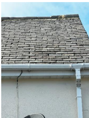
Pic 8: mis aligned ridge tiles
