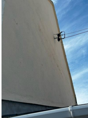
Pic17: Damaged render
