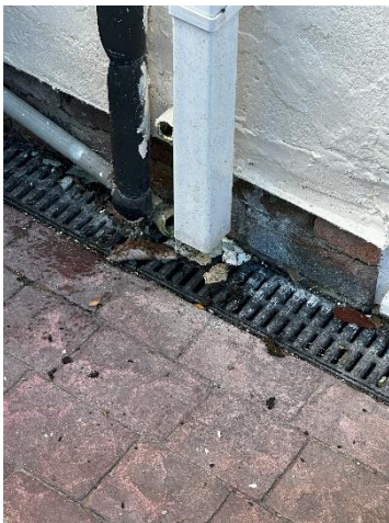
Pic12: down spout cut short of gulley
