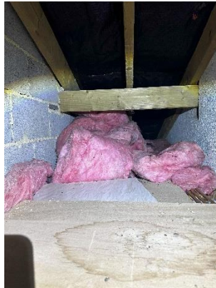
Pic27: displaced insulation
